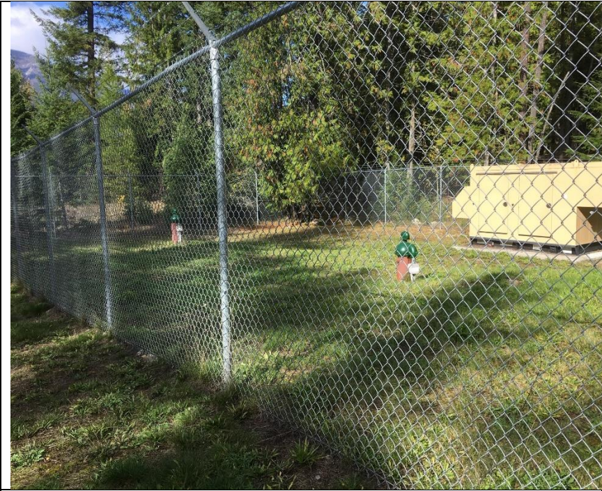
Fenced Enclosure for Well Heads
