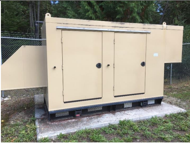
Onsite Diesel Generator
